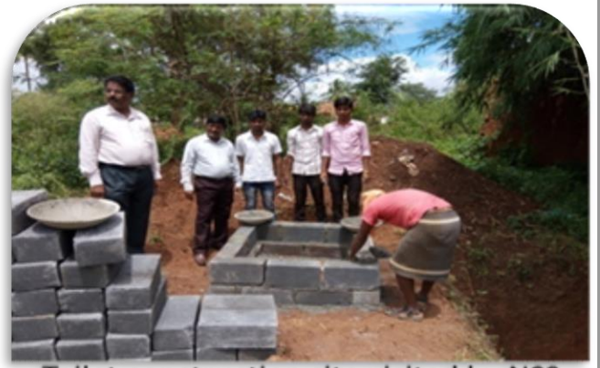
Toilet construction site visited by NSS Program Co-ordinator Dr. M. B. Dalapati.
