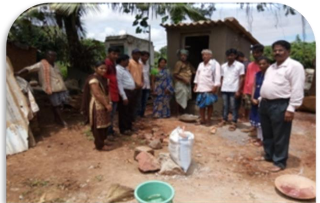
Toilet construction site visited by NSS Program Co-ordinator Dr. M. B. Dalapati.
